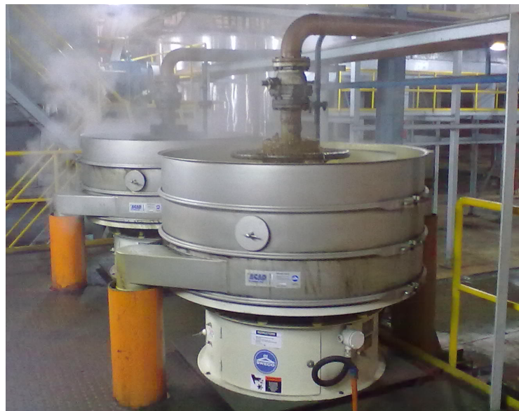
Fig 1. Double Deck Vibrating Screen
