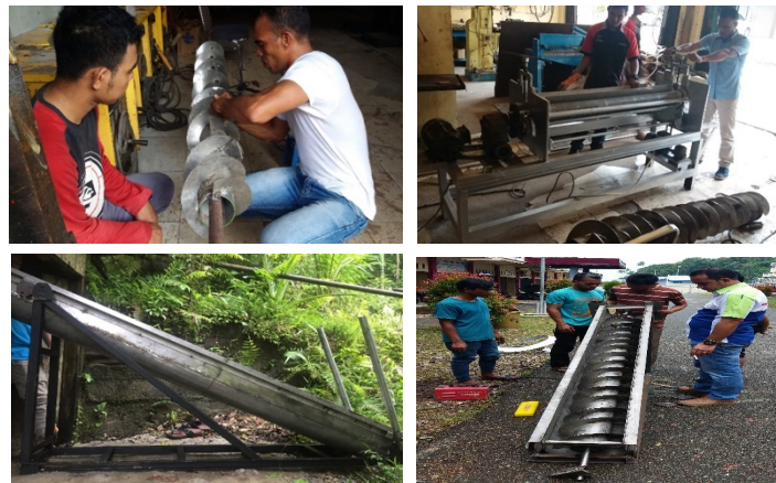
Fig. 7. Manufacture Archimedes Double Screw Turbine
