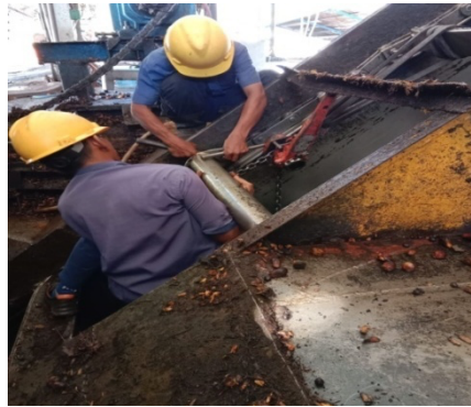
Fig. 3. Failure Analysis on Conveyor Scrapper
