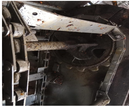
Fig. 2. Chain Conveyor Scrapper
